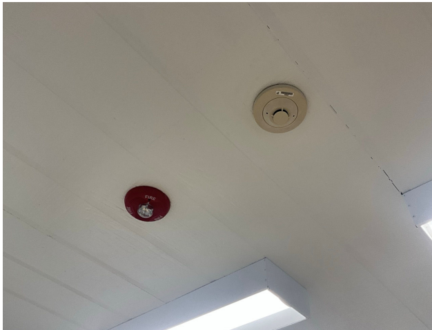
39 - FIRE ALARM SYSTEM
