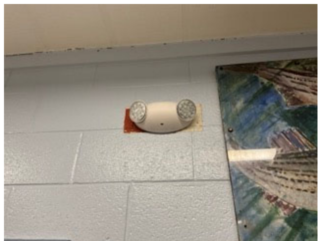
36 - EMERGENCY AND EXIT LIGHTING SYSTEM
