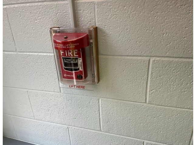
38 - FIRE ALARM SYSTEM
